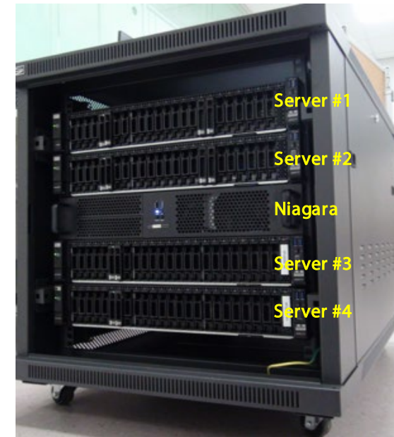
[Rack-Scale System with Niagara]
