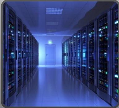
SW Defined Datacenter
